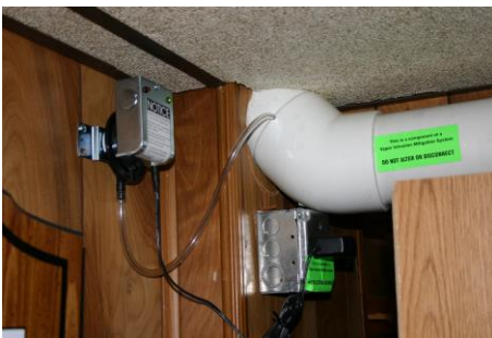
Audible alarm and system labels
